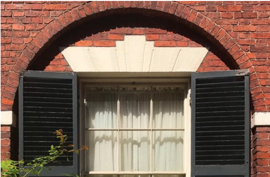
Exterior of Nichols House Museum showing Flemish bond, recessed arch, lintel, and stringcourse.
