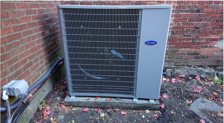
Upgraded air-cooled condensing unit for floors one through three of the Museum.
