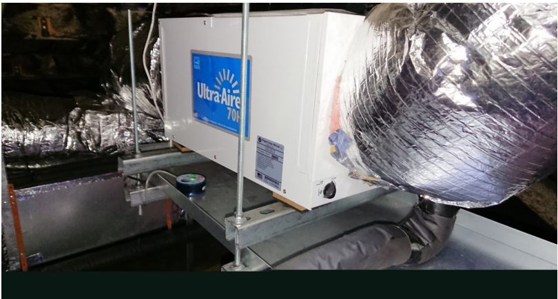
One of two side-stream dehumidifier units, this one in the attic servicing the archive and collections storage area.
