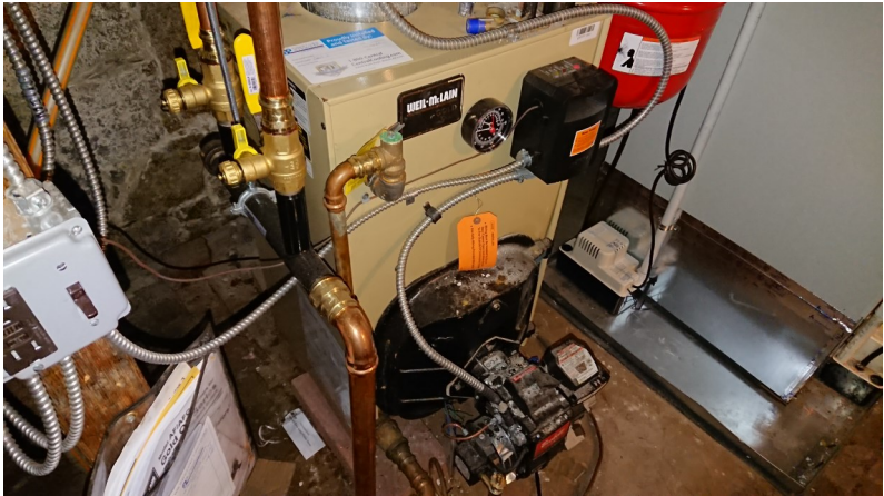
Weil-McLain cast iron boiler installed in basement.
